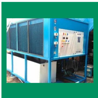
45 TR Water Cooled Chiller
