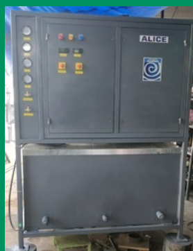
20 TR Air Cooled Brine Chiller
